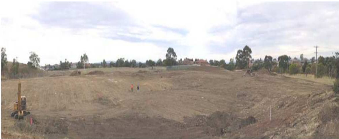
Figure 2. Panorama of depressed central area during preliminary site stripping (Avalue and McKenzie, 2005).
